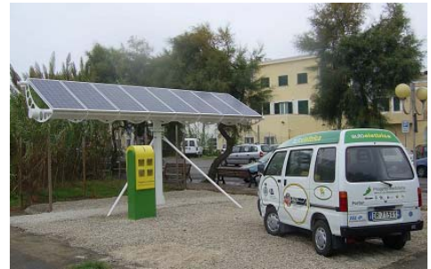
Figure 5: The integrated photovoltaic charging station.
